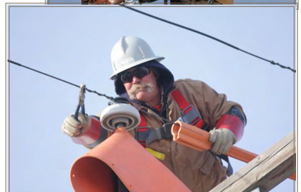
Journeyman Power Line Technician applies “cover up” in order to execute rubber glove work procedures.
