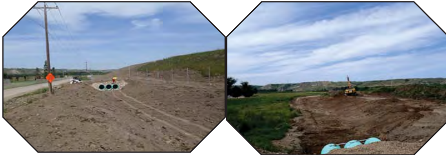
Aligning of culverts allow for the better flow when storm water passes.
