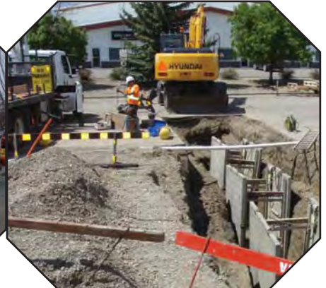
A new water service installation 1600 Blk. - 36 Street North (shoring being used to protect workers while working in the trenches)
