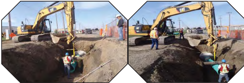
This installation required a lot of care as the pipe had to be installed below ATCO gas line.
