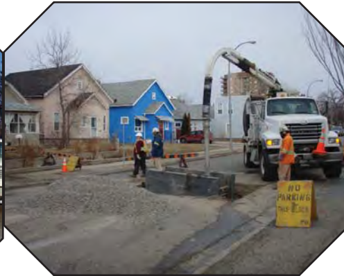
Hydro-vac vac exposing a water service leak at the watermain in the 600 Block. - 7 Street South
