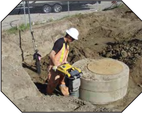
Compacting soil around a Manhole installing a sanitary service 4000 Block 2 Avenue South
