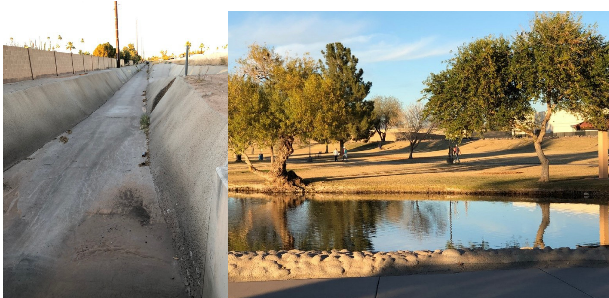
FIGURE 2.6 (Left) A concrete channel in Scottsdale, Arizona. (Right) Indian Bend Wash Greenbelt. SOURCE: Photos courtesy of Lauren Alexander Augustine, the National Academies.
