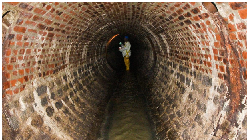
FIGURE 1.1 Brick sewers built in Philadelphia, some of which are nearly 200 years old, are still in use today. SOURCE: Photograph by Kimberly Paynter.
