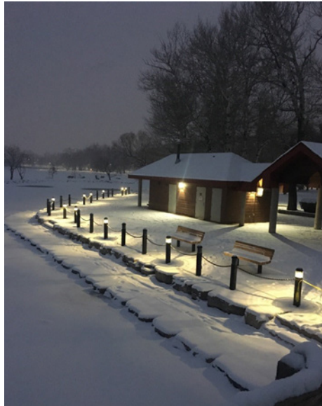
Henderson Lake Park Lighting
